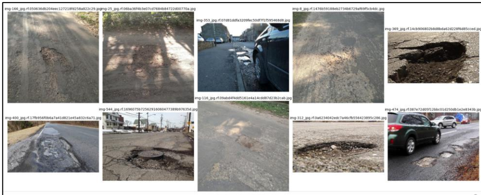
Fig. 2 – Examples of road potholes in diverse conditions.
