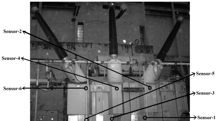
Fig. 3 –View of 250 MVA 15.75 kV/420 kV generator transformer with sensors mounted (sensors mounted on the HV side of transformer tank are seen).
